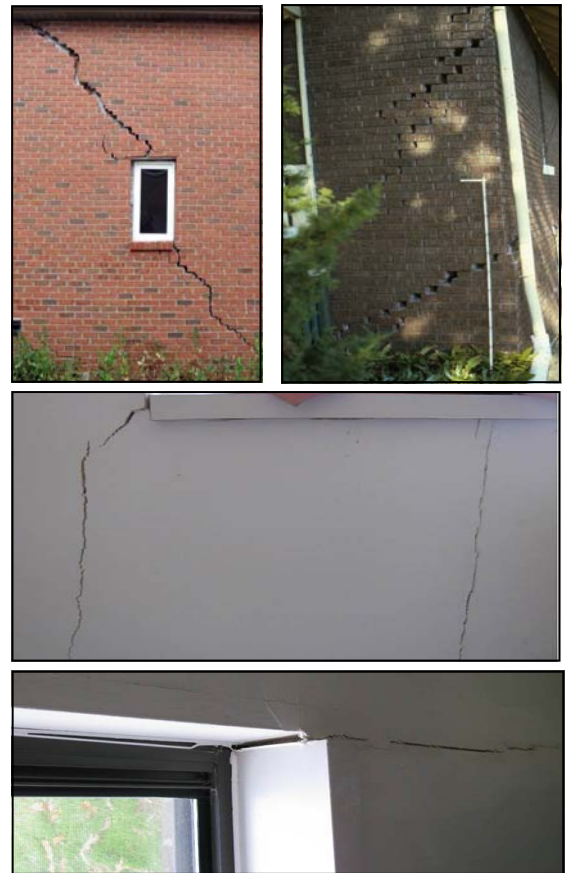
FIGURE 1 EXAMPLES OF AESTHETIC DAMAGE
