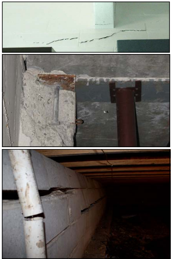
FIGURE 3 EXAMPLES OF STRUCTURAL DAMAGE
